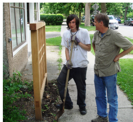
Nik, left, with his mentor, Alphonse, in front of the store with the completed outdoor wall they built with a Japanese tongue and groove technique.
